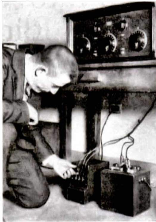
Fig. 3— Simple installation of a B battery eliminator. Simply connect wires between the binding posts of the radio receiver and those of the eliminator, and plug the eliminator into wall socket. At right is seen the A battery. A cable holds all leads for battery and eliminator.
